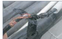
Cases of field defects
